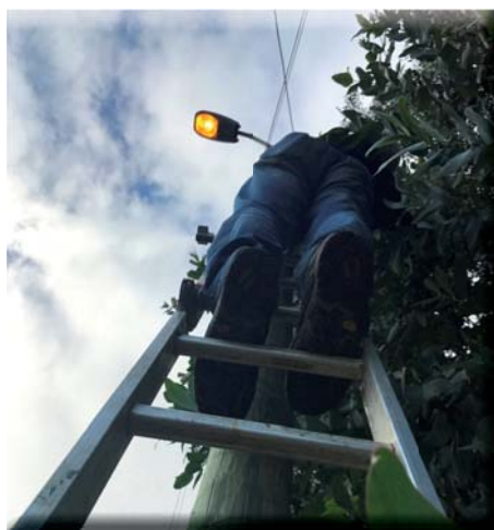
Checking the lamps outside of the bungalow
